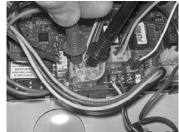
Checking MV & MV/PV control plug pins to gas valve for 24 volts output during heating cycle (pilot must be lit with no sparking).
