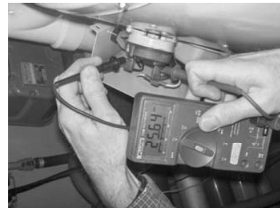
Checking pressure switch contacts. Contacts are open if blower is operating and there is 22-26 volts measured between the two contacts (as in photos)
