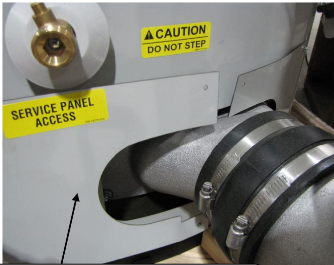
Exhaust tube pressure tap located behind service panel access doors at bottom of heater
