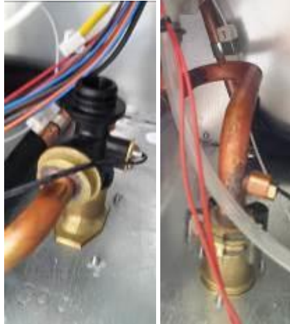
Figure 29 – Outlet Water Temperature Sensor (left) and Inlet Water Temperature Sensor (right)
