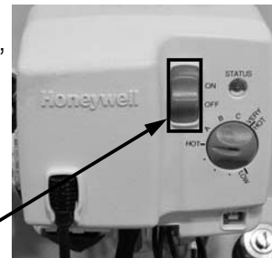
Gas control power switch
