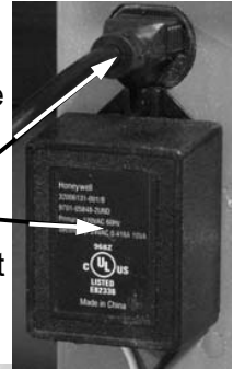
Water heater power cord and Accessory Module transformer
