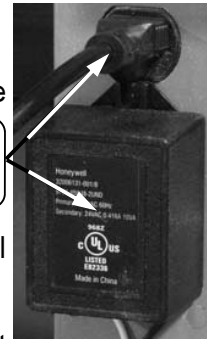
Water heater power cord and Accessory Module transformer
