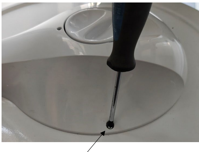
Fig. 2a Junction Box
