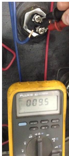
Figure 14. Resistance Check of Element using a Multi-Meter
